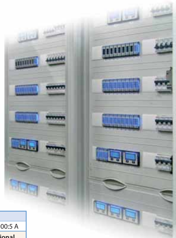
A large number of energy meters in the smallest of spaces ►
