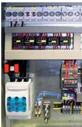
▲ Current converter in switch cabinet
